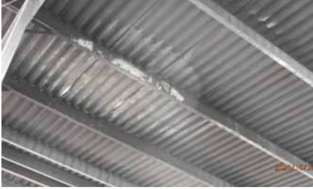
Figure 5 - Damaged Roof Area
