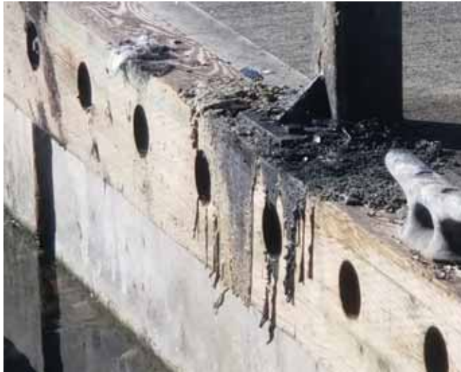
Figure 6 - First Damaged Column
