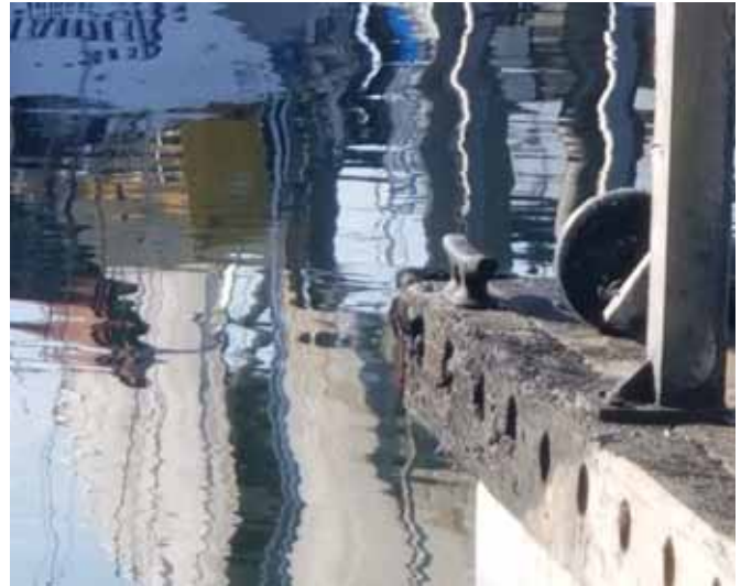
Figure 7 - Second Damaged Column
