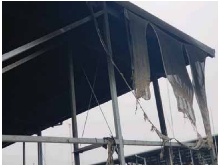
Figure 8 - Damaged Fire Curtains
