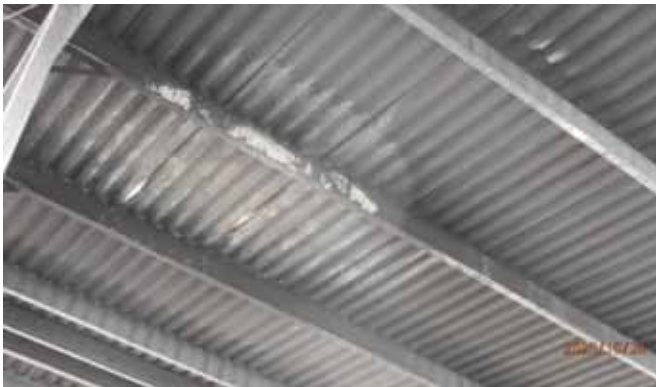
Figure 4 - Damaged Roof Area
