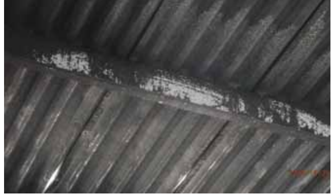
Figure 6 - Purlin Galvanizing Damage
