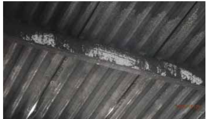
Figure 5 - Purlin Galvanizing Damage
