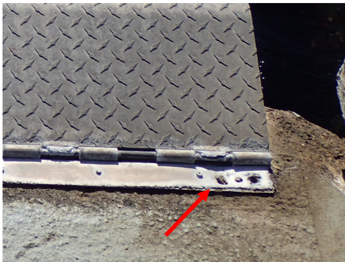
Photo S2.3-9: Missing Transition Plate Anchors
