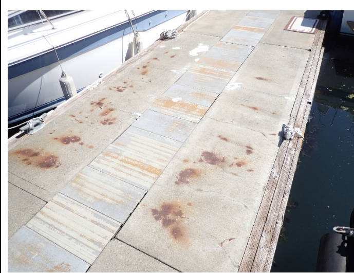
Photo S2.4-7: Delaminated Concrete and Rust Staining in Float Modules at Mid-Point of Service Float
