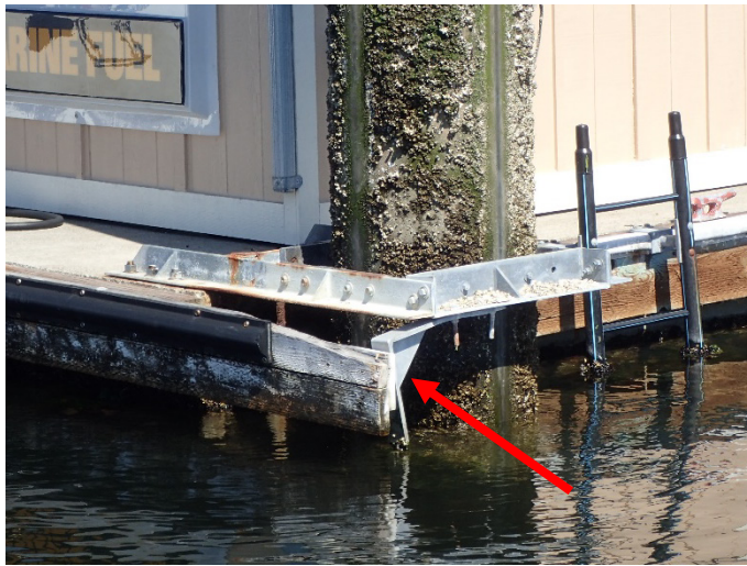
Photo S2.4-14: Failed Guide Pile Assembly Bracket on South End of West Breakwater
