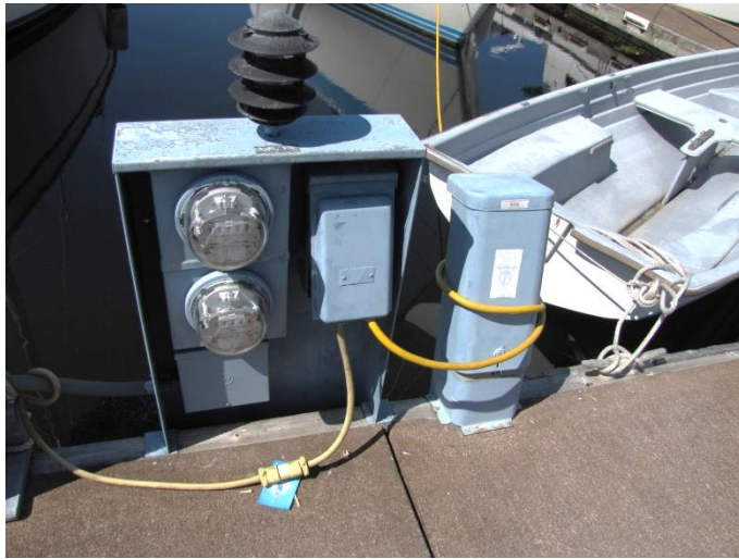
Photo E2.1-1: Typical A dock powercenter
