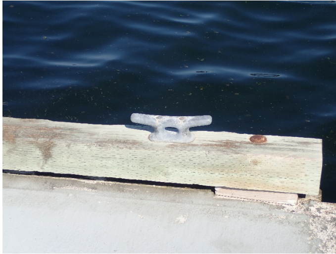
Photo S2.2-7: Typical Galvanized Steel Cleat Condition
