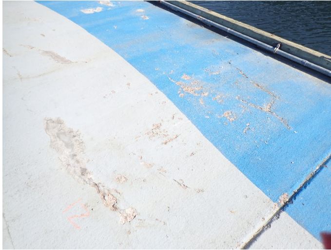
Photo S2.3-4: Delaminated Concrete in Top of Deck Surface
