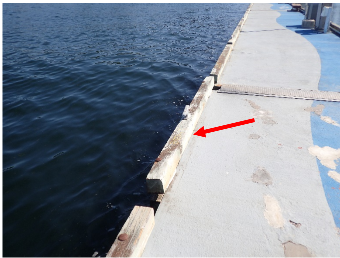
Photo S2.3-11: Displaced Timber Curb With Bent Anchor Bolts
