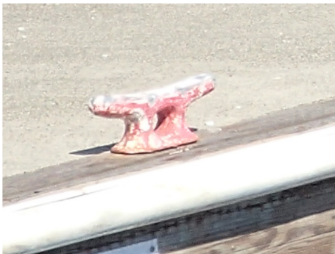
Photo S2.4-9: Typical Coated Cleat Condition
