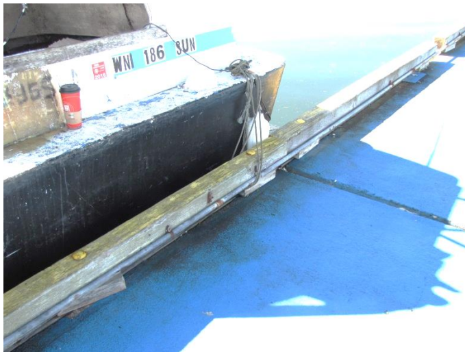
Photo E2.3-2: Ship tied to curb and conduit, subjecting conduit to possible mechanical damage
