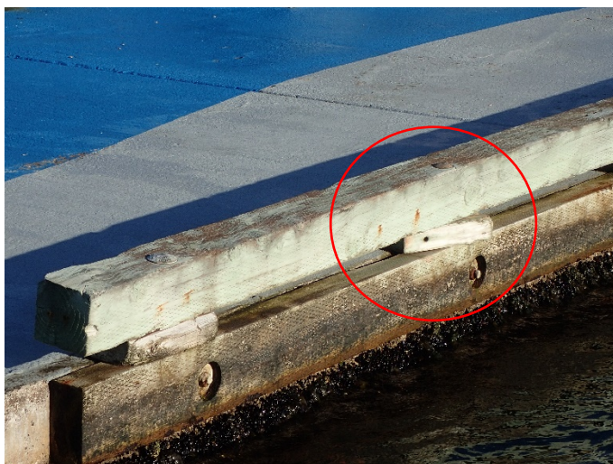
Photo S2.2-12: Typical Loose Timber Curb and Spacer Blocks
