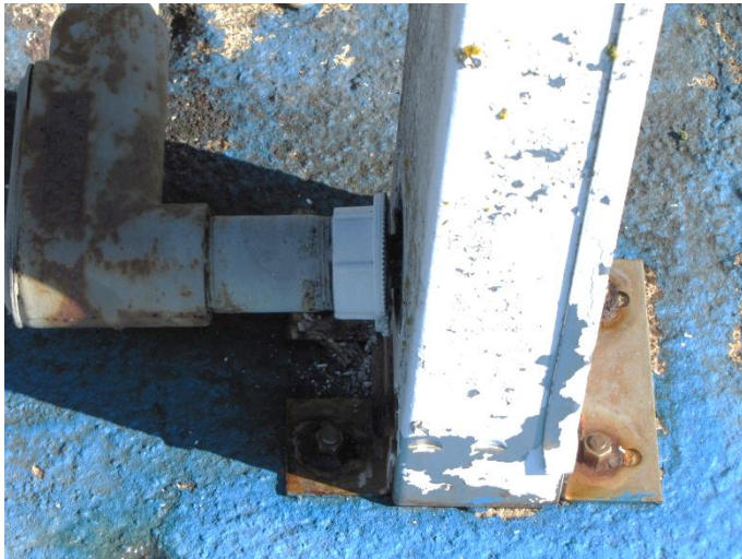
Photo E2.2-2: Powercenter pedestal with rusted angle brackets, rusted bolts, loose connection fitting and rusted conduit
