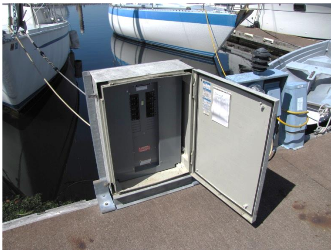
Photo E2.1-6: Panelboard A3 (A2 similar)
