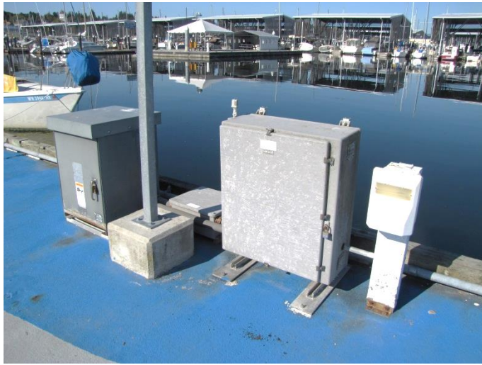
Photo E2.2-4: Typical transformer, splice box, panelboard, light pole and powercenter
