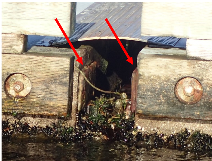
Photo S2.2-11: Typical Corrosion of Steel Connection Hardware
