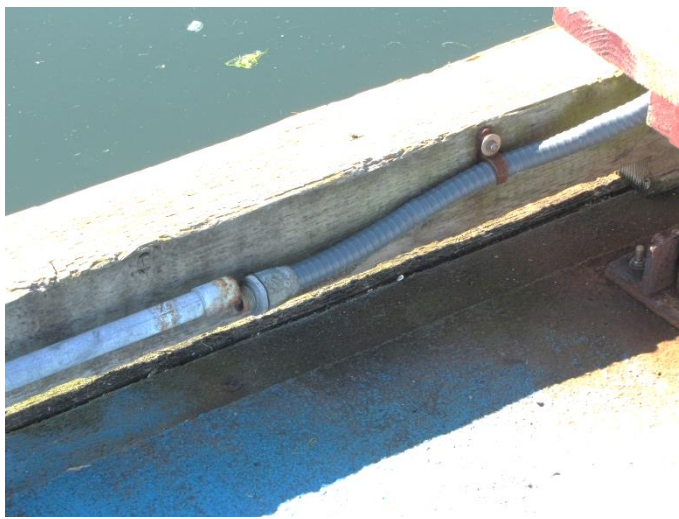
Photo E2.3-1: Detached conduit fitting
