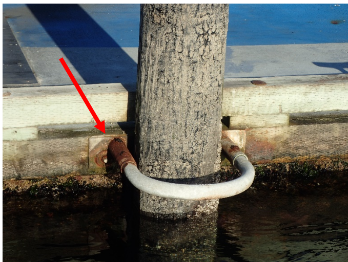
Photo S2.2-9: Corrosion on Steel Pile Guide Assembly
