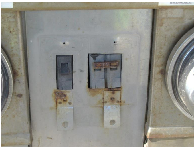
Photo E2.4-3: West end powercenter with missing covers on circuit breakers
