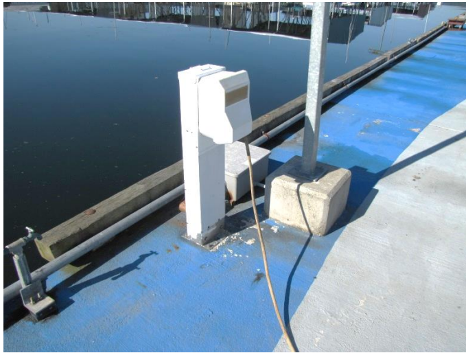
Photo E2.3-10: Typical powercenter, splice box and light pole with power cord draped across breakwater.
