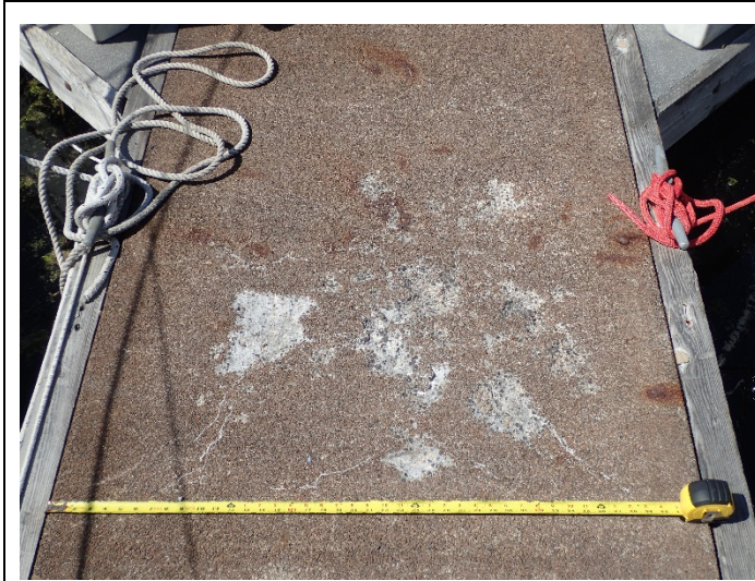
Photo S2.1-4: Cracking, rust staining, and surface spalling in concrete float module
