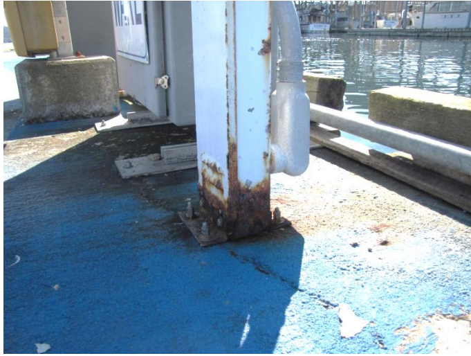
Photo E2.3-7: Rusted powercenter pedestal, angle bracket
