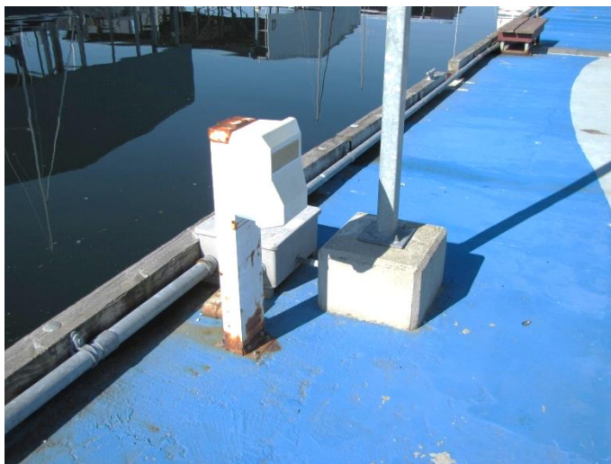
Photo E2.3-6: Powercenter with rusted pedestal, conduit and angle brackets
