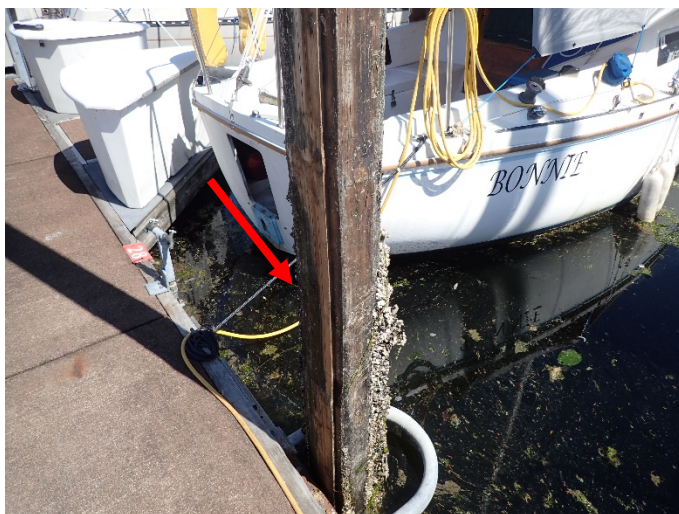
Photo S2.1-3: Moderate abrasion and section loss in timber guide pile
