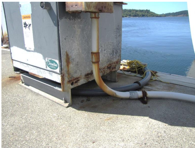
Photo E2.4-5: Rusted transformer #2
