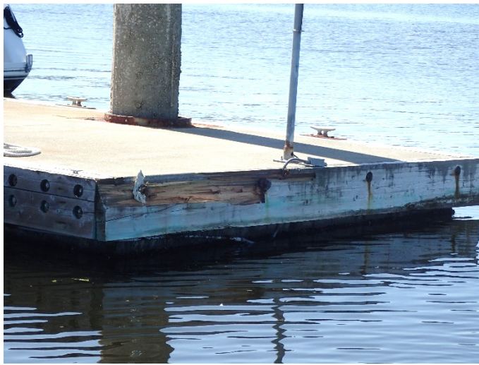
Photo S2.4-11: Failed Timber Rub Strip at North End of West Breakwater
