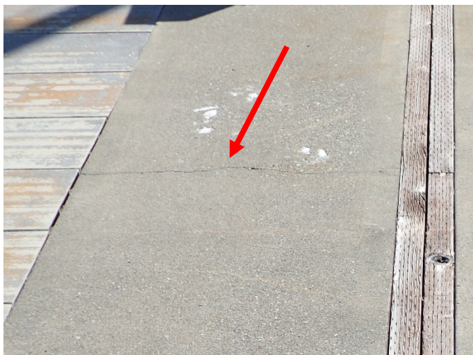
Photo S2.4-6: Typical Cracking in Service Float Modules
