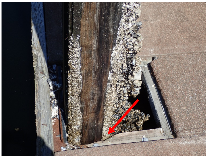
Photo S2.1-8: Typical worn pile guide assembly rub block
