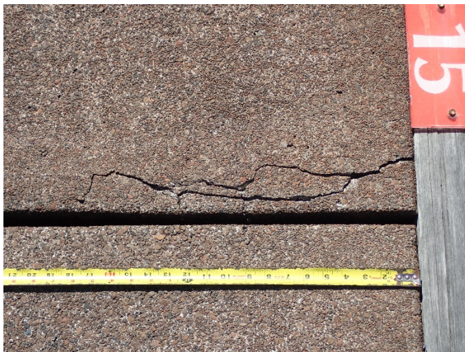
Photo S2.1-5: Delamination in concrete float module
