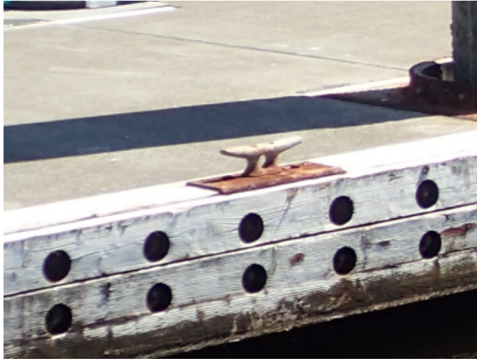
Photo S2.4-10: Steel Cleat on West Breakwater with Corrosion and Scaling on the Base Plate
