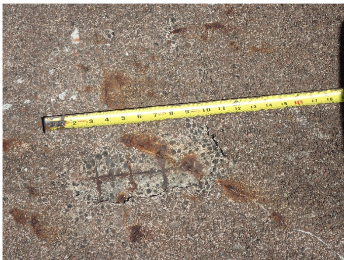
Photo S2.1-6: Spall with exposed reinforcing steel in float module, note abraded concrete surface.
