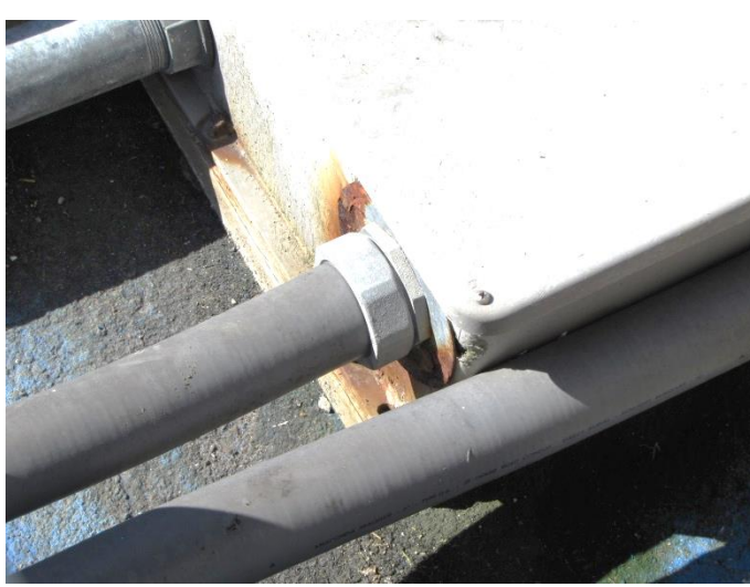
Photo E2.3-4: Previously repaired portion of damaged splice box with new rust
