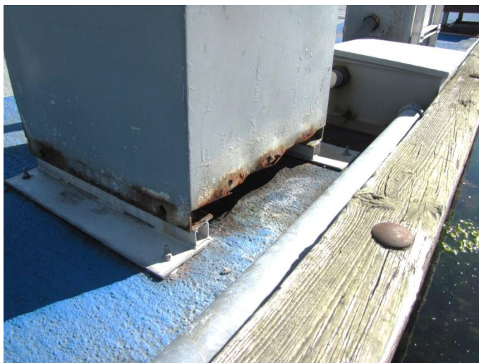
Photo E2.3-12: Rusted transformer bottom
