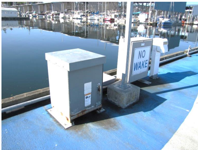
Photo E2.3-11: Typical transformer, splice box, light pole, panel and powercenter.
