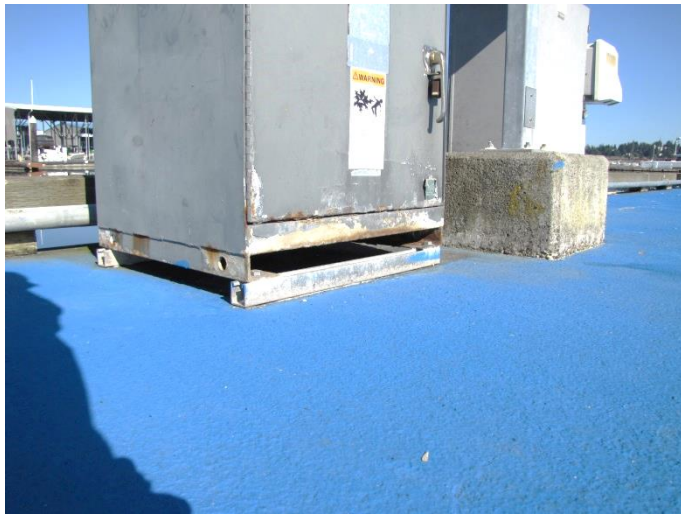
Photo E2.2-5: Transformer with rusted bottom
