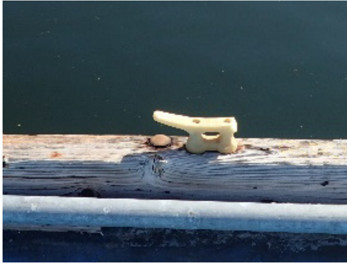
Photo S2.3-7: Broken Cleat
