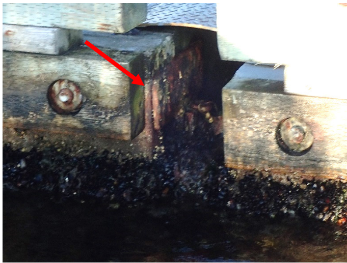
Photo S2.3-10: Typical Corrosion of Steel Connection Hardware
