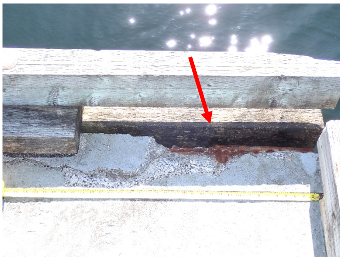
Photo S2.3-6: Open Corrosion Spall with Exposed Reinforcing
