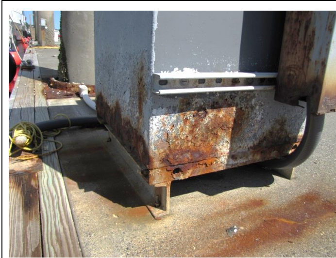
Photo E2.4-4: Rusted transformer #2
