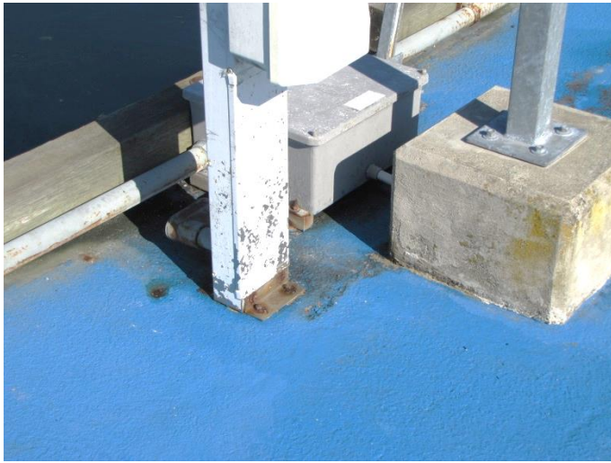
Photo E2.2-1: Typical powercenter, splice box and light pole
