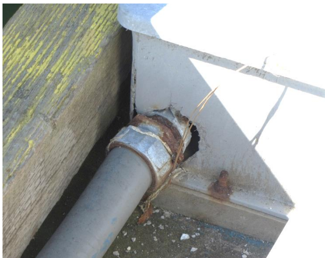
Photo E2.3-3: Damaged splice box
