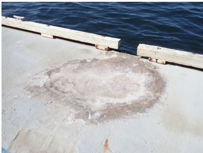
Photo S2.3-5: Previous Repair in Top of Deck (Minor Edge Delamination)
