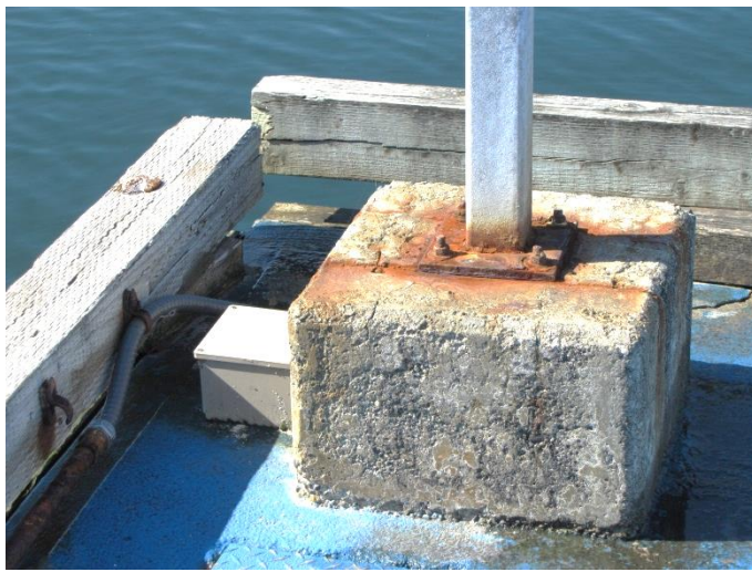
Photo E2.3-5: Rusted beacon pole footing, conduit not mounted to curb
