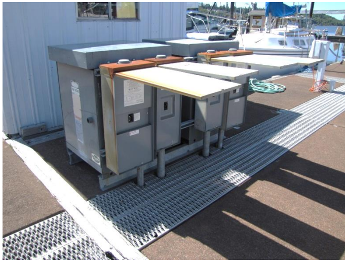
Photo E2.1-5: Transformers TRA2 and TRA3 with enclosed circuit breaker covers open
