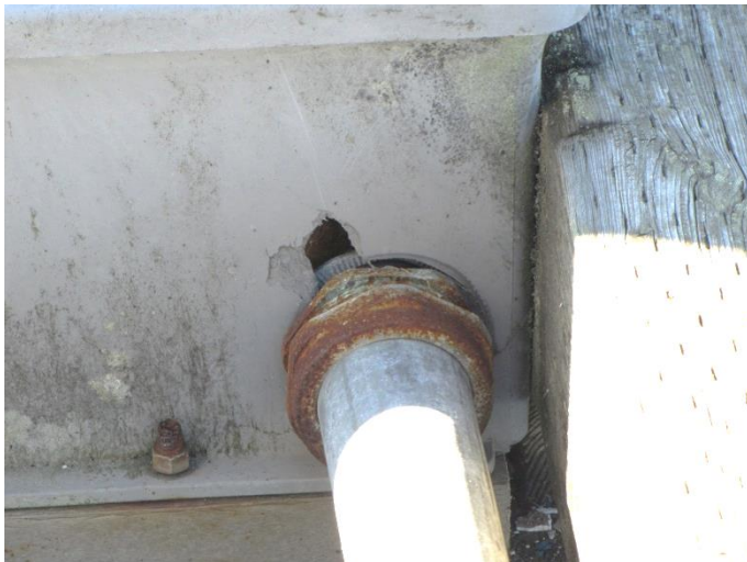
Photo E2.2-3: Broken splice box, rusted fitting, rusted bolt
