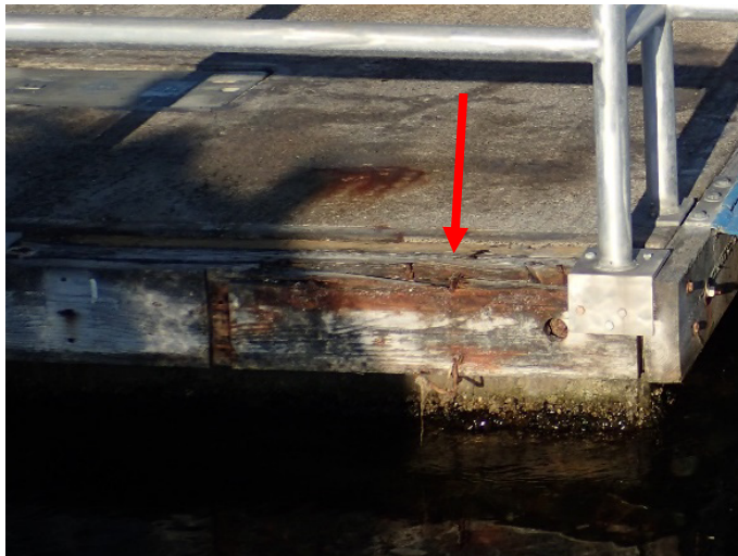
Photo S2.2-8: Fungal Decay in Timber Rub Strip at Northeast End of Approach Floats
