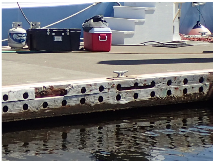
Photo S2.4-12: Failed Timber Rub Strip 20' from North End of West Breakwater
