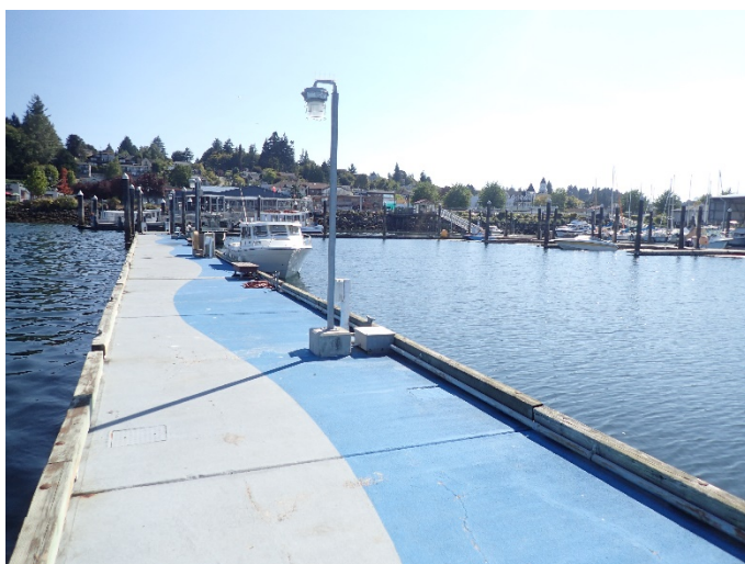
Photo S2.2-6: Typical Condition of Concrete Breakwater Float Modules (Looking Southwest)
